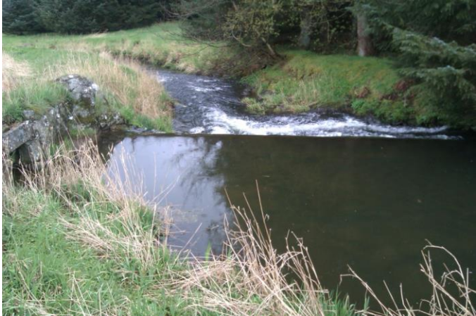
Bronie Scottiesly Weir May 2012, looking downstream. (Note the location of the unused lade take-off on the left of the picture.)
